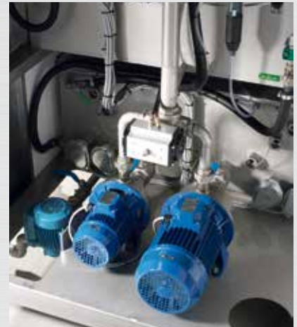
Easy access to the system, pumps etc.
